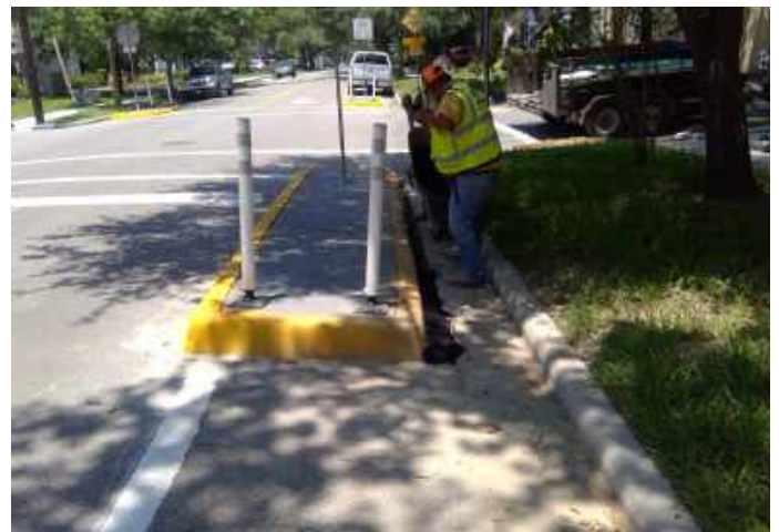
Pavement patching next to newly installed bulbout (punch list item)
